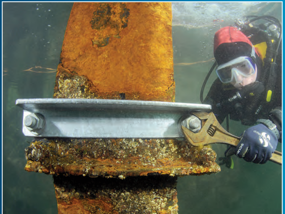
NFSD diver replacing retaining brackets on one of the UK tide gauges.
